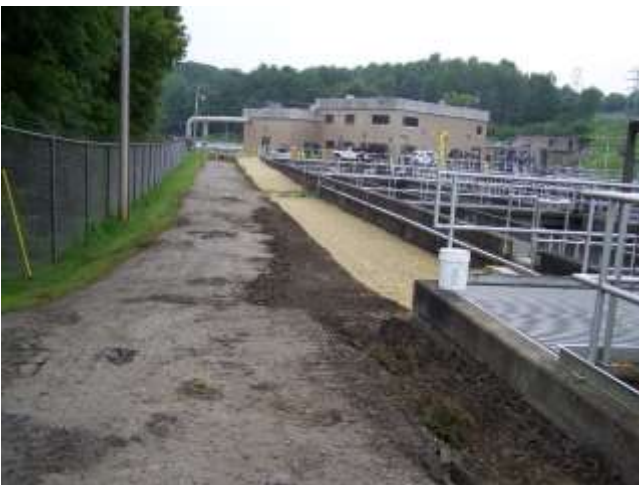
UV Disinfection Buried Electrical Cables
