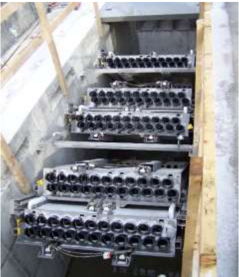
Banks of Installed UV Tube Modules
