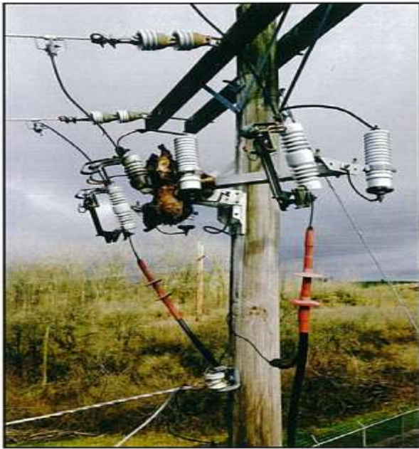
Large raccoon climbs utility pole and trips out a sewage treatment plant.
