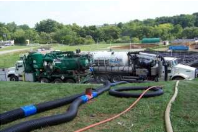
VAC Trucks outside Secondary Digester
