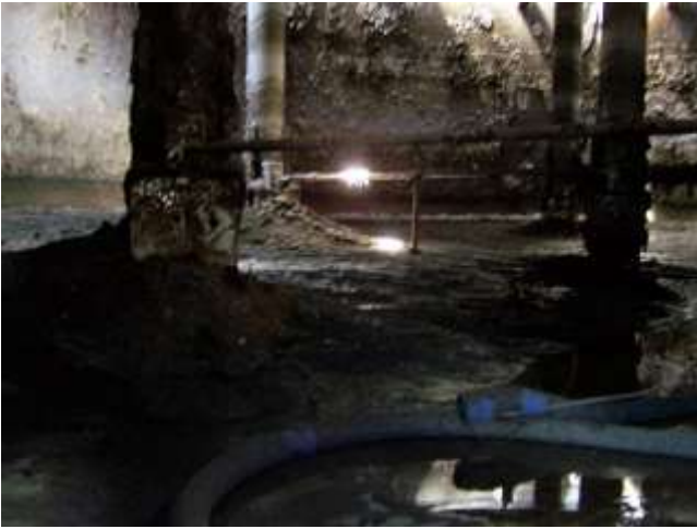
Grit inside Primary Digester
